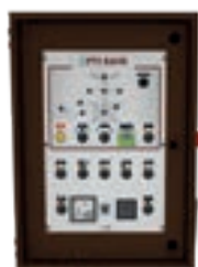
Armoire Opti Rain Opti Rain Control box
